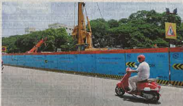
A quiet start: Barricades have been placed at several places as part of the Metro phase II project. ■SPECIAL ARRANGEMENT
