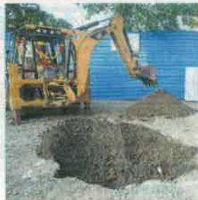
The foundation stone being laid for the Metro phase II at Villivakkam. ■ K. PICHUMANI
