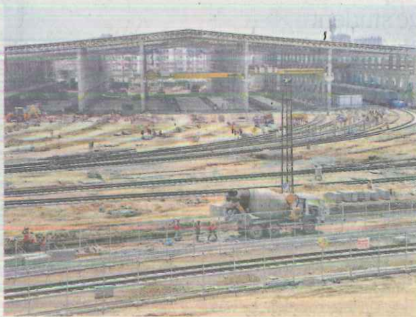
Maintenance hub: Depots are crucial for the everyday upkeep of the metro trains. ■ FILE PHOTO
