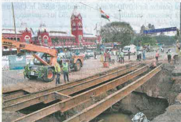
Restoring normalcy: The caved-in deck on E.V.R. Salai near Central station being repaired on Monday. ■ S.R. RAGHUNATHAN
