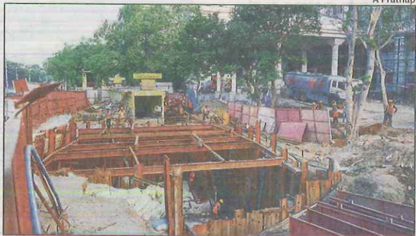
PEDESTRIAN FACILITY: Subway construction work on near the Rajiv Gandhi Government General Hospital on Thursday
