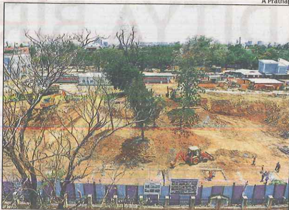
CMRL carries out construction of a parking area and amenities centre at Thiru Vi Ka park in Shenoy Nagar
