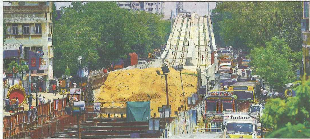
TAKING SHAPE: The ramp (above) that will link the underground section to the elevated corridor near Tondiarpet will be completed by June next year. The elevated corridor being built near Tiruvottiur
