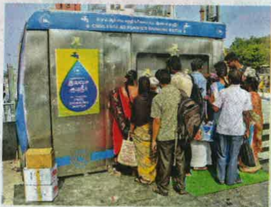
The RO plant at Central Metro Rail station offers drinking water for free to the public
