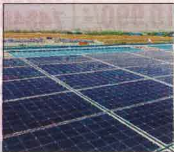
GREEN ENERGY: A solar power plant at one of the two metro stations
