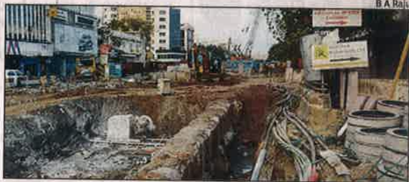
Construction of one of the two entry points for Thousand lights metro station underway on the day of inauguration in February
