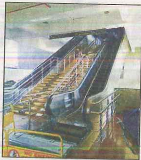
The new escalator being installed will help passengers headed to the airport
