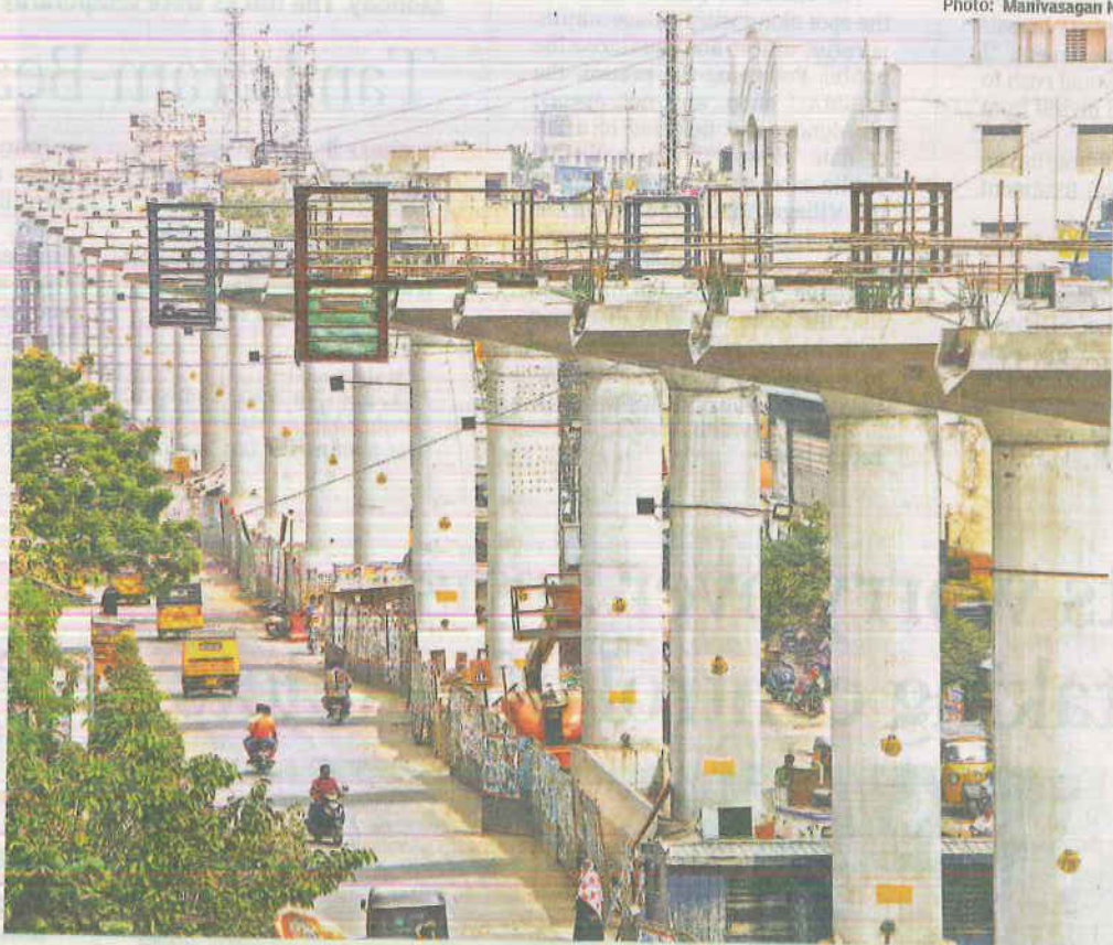
STANDING TALL The Metro connectivity is getting increasingly better with more areas coming under its cover. Here, the pillars have been erected at Tiruvottiur, where the Metro is expected to decongest the roads
