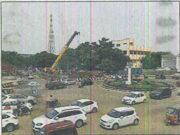
PEDESTRIANS FIRST: Work is underway to excavate soil at the intersection to build the subway at the roundtana in Anna Nagar
