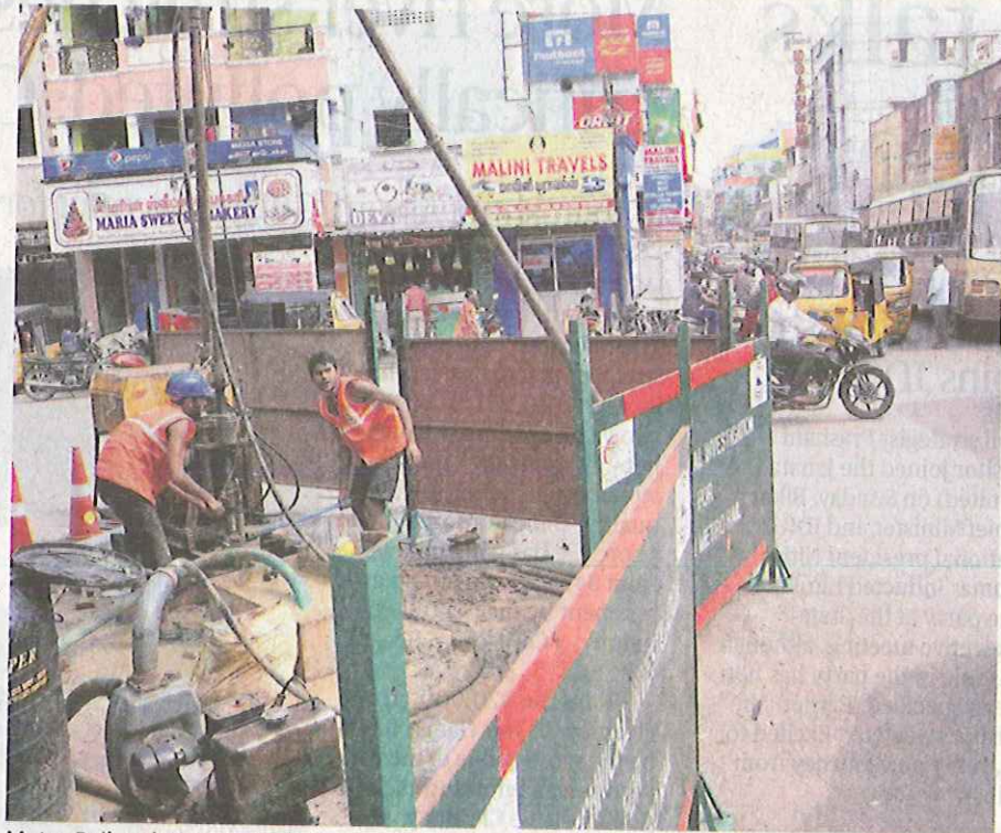
Metro Rail technicians putting up scaffoldings for soil testing work on the Perambur Barracks Road recently. ■ B. JOTHI RAMALINGAM
