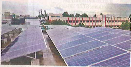
Solar panel installed at Anna Nagar East station
