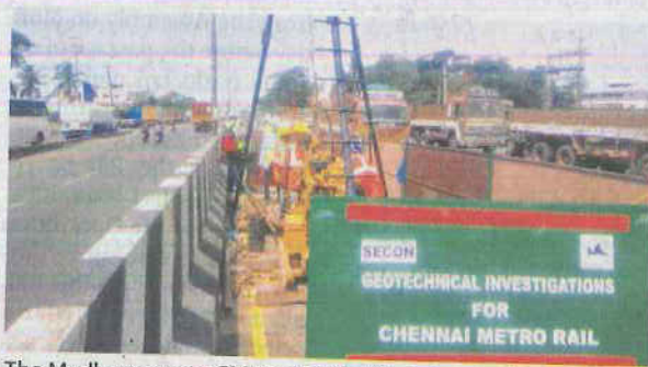
The Madhavaram to CMBT and the Madhavaram to Sholinganallur stretches will be constructed at a cost of ₹44,000 crore. ■ B. JOTHI RAMALINGAM
