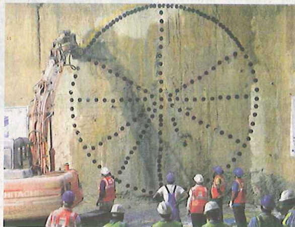
All set: The tunnelling work on the Anna Salai stretch got over recently. ■ FILE PHOTO
