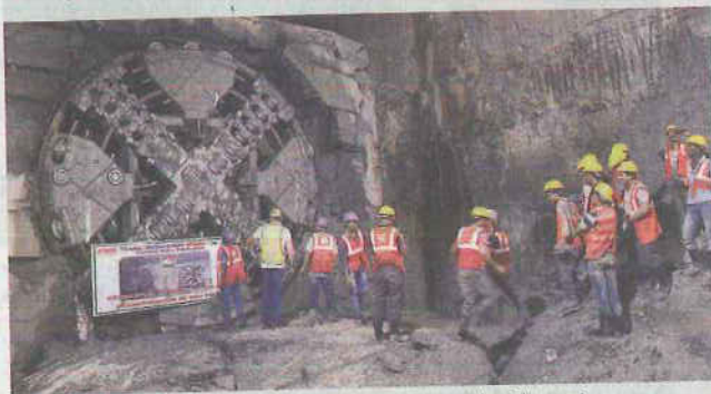
Moving ahead: Tunnelling work in progress at the Chennai Central metro station. ■ R. RAVINDRAN
