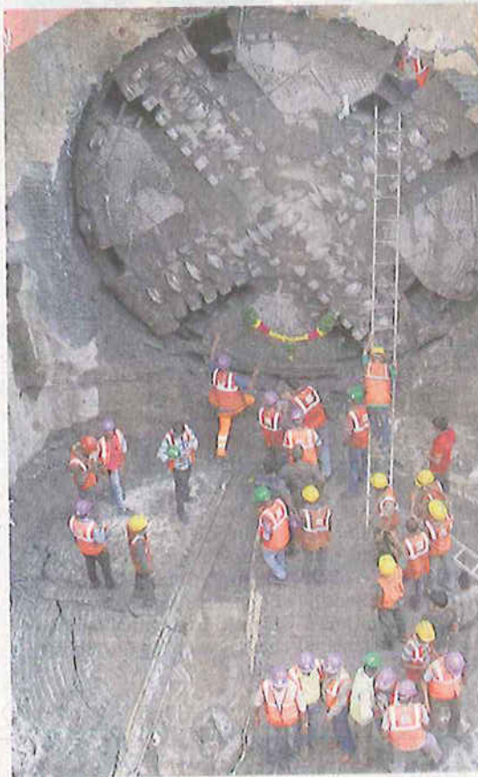
On the right track: The tunnelling work for phase I extension – from Washermanpet to Korukkupet – was completed recently, nearly a year after it began. •FILE PHOTO
