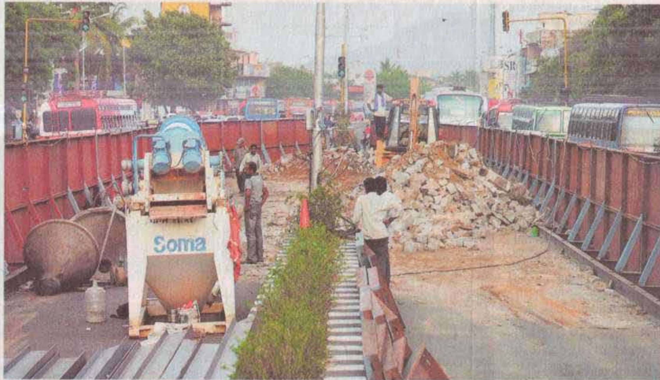
CRUCIAL CHECK: Soil testing for the Metro Rail project under progress on 100 Feet Road near Koyambedu on Monday. - PHOTO : K. PICHUMANI
