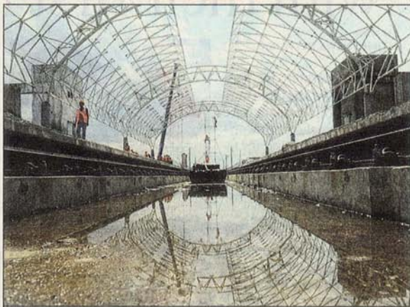
The signals have been installed at Koyambedu depot (above)
