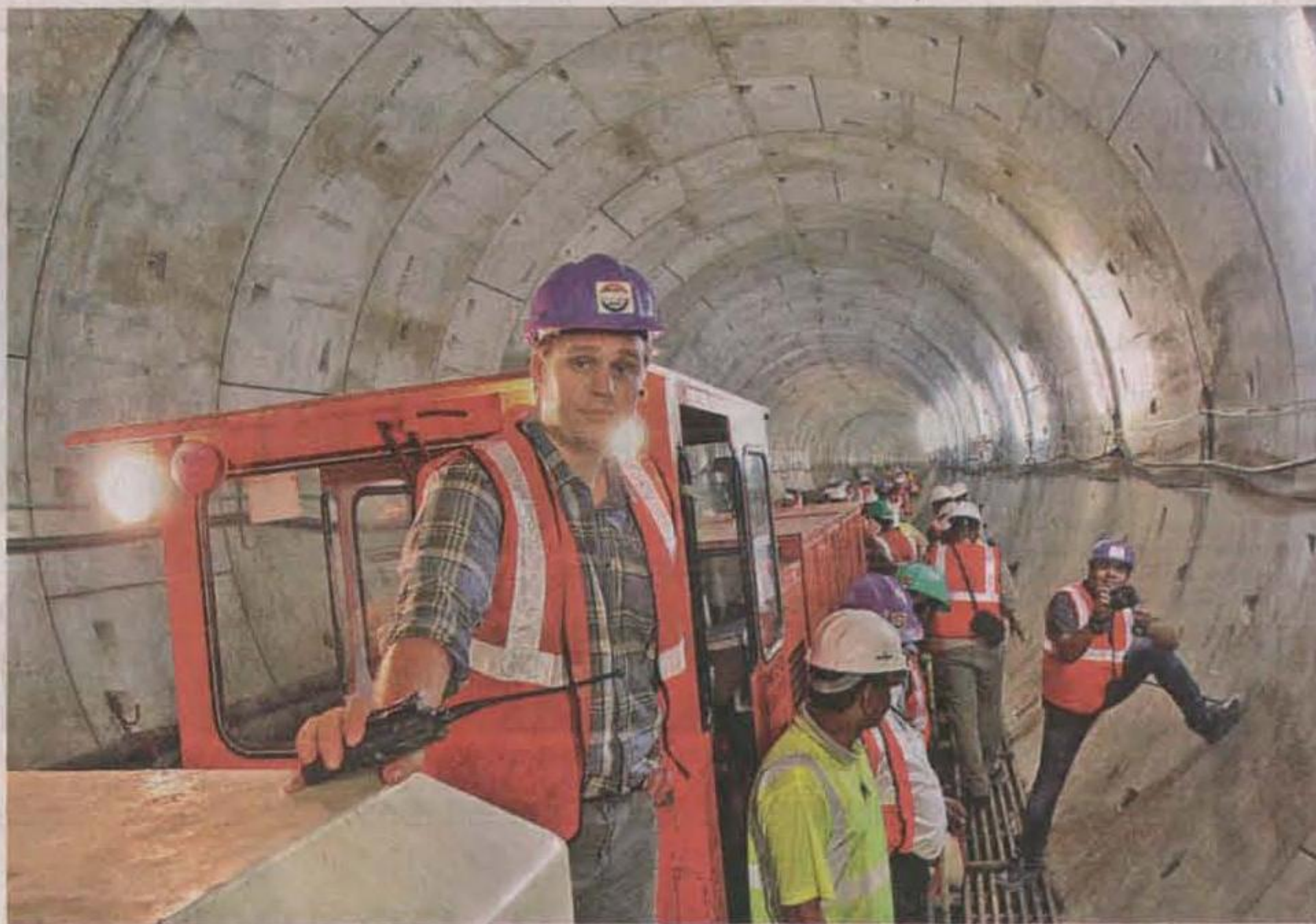
A view of the tunnel leading to Anna Nagar Tower station from Shenoy Nagar.
