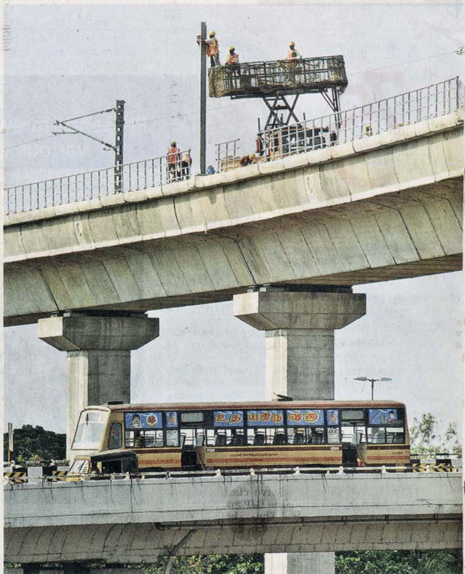
Electrical works going on at the metro rail bridge above Kathipara flyover.
