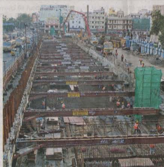
A row of iron beams shows extent of strutting done to support the underground station works near Central.
