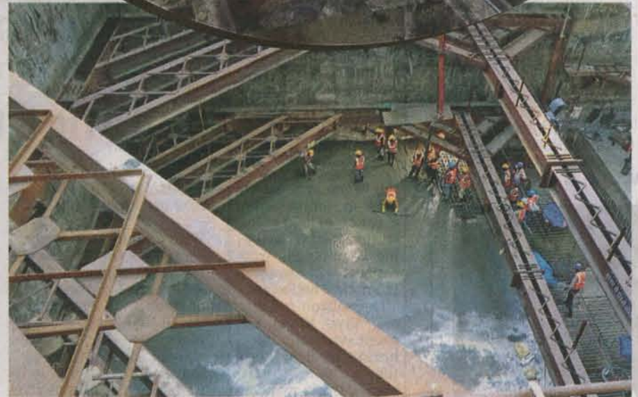
At Thirumangalam, workers are busy finishing the base slab while iron beams hold the diaphragm walls together.
