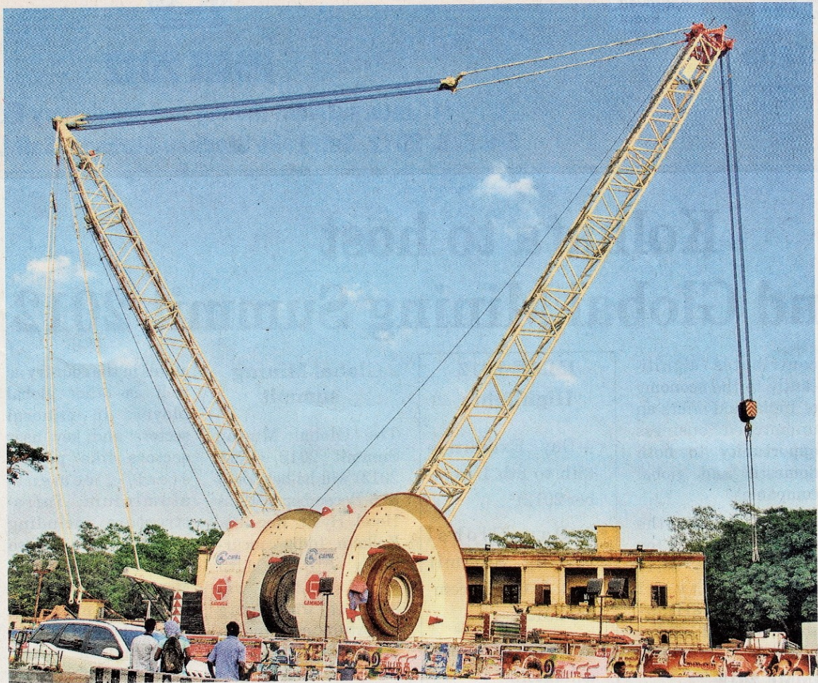
Gaining pace: Heavy machinery in place for the Chennai Metro Rail work at Saidapet, Chennai. — Bijoy Ghosh
