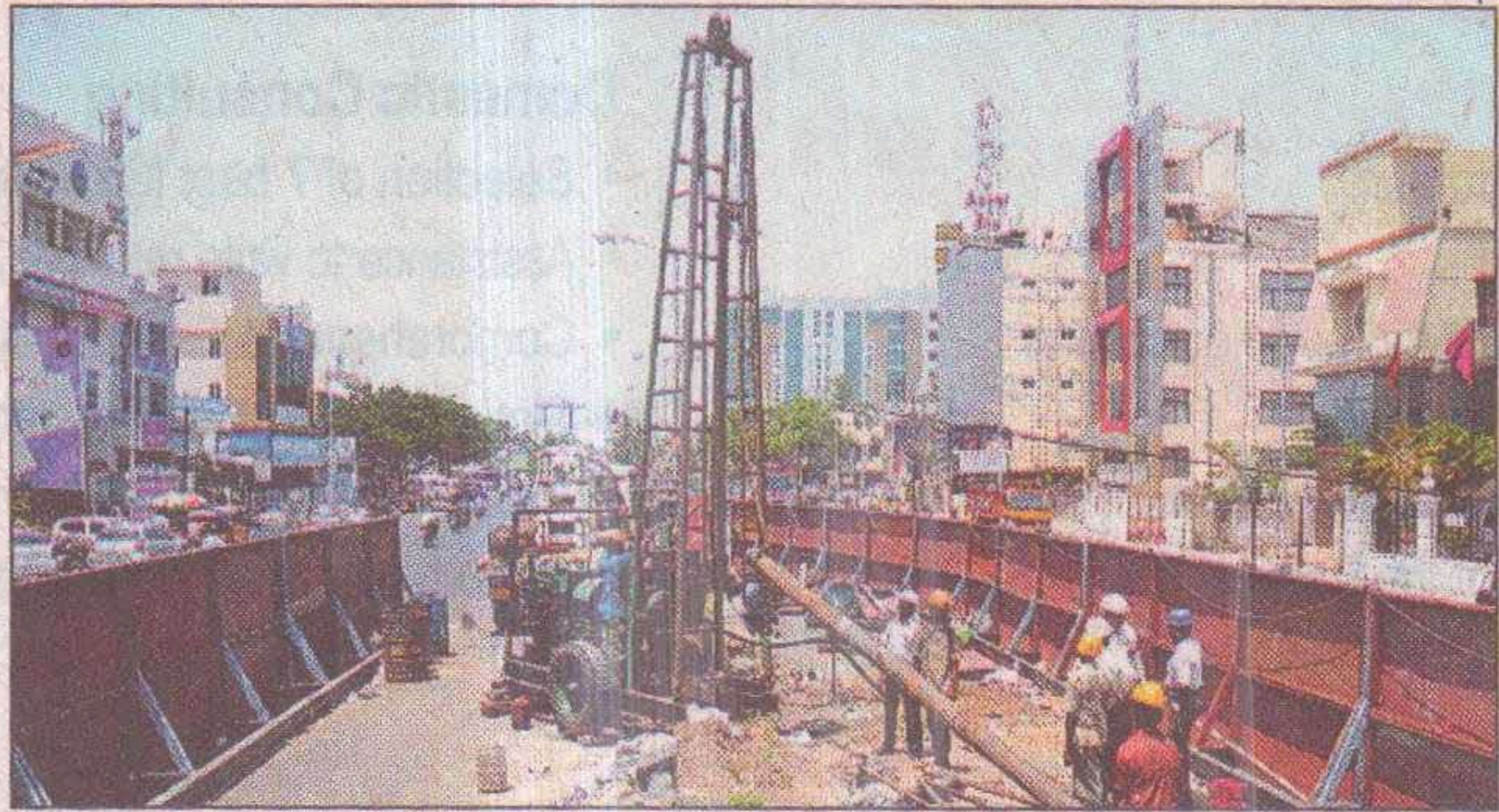
BRISK PACE: Soil testing for Metro rail project being done near Ambika Empire Hotel in Vadapalani
