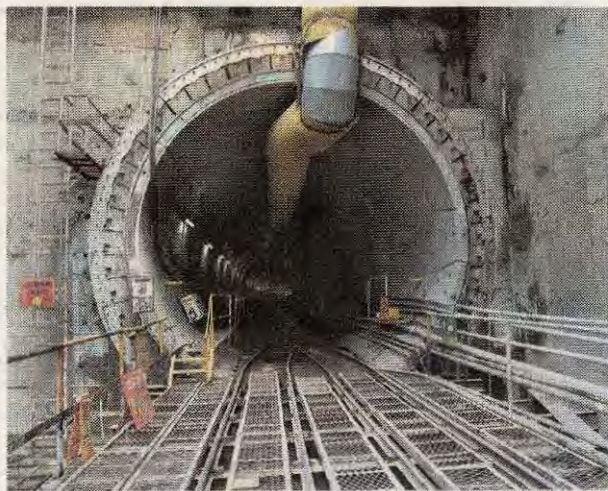
CMRL is ensuring safety exits for commuters taking the underground metros | EXPRESS
