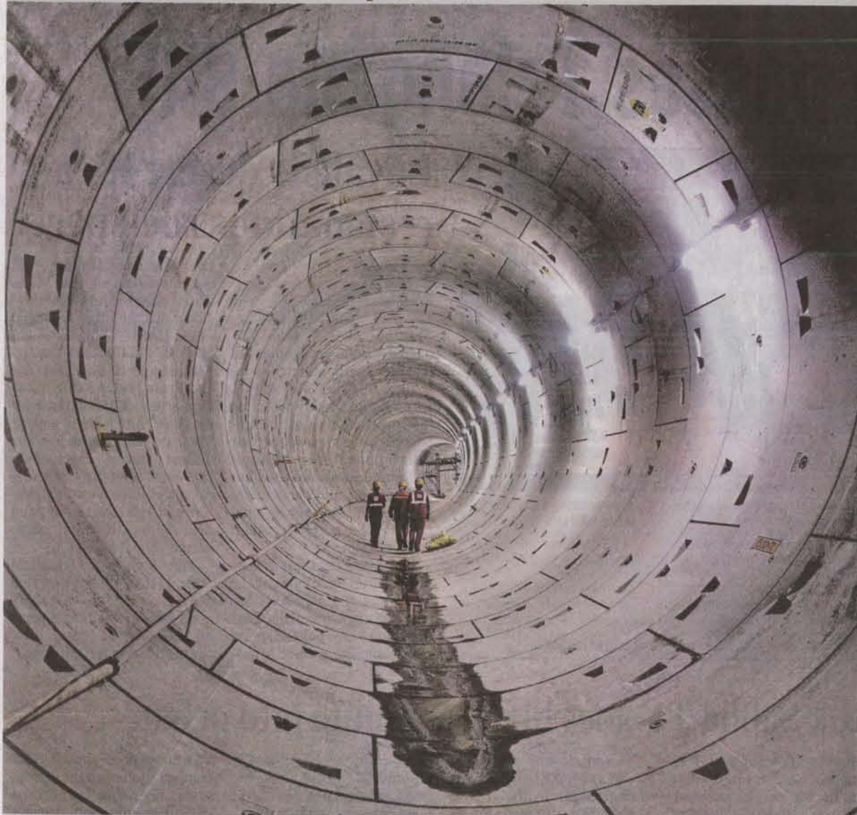
Two tunnel boring machines from China were employed to drill from Nehru Park to Egmore and it took nearly 18 months for the machines to tunnel a distance of about 950 metres — PHOTOS: S.R. RAGHUNATHAN
