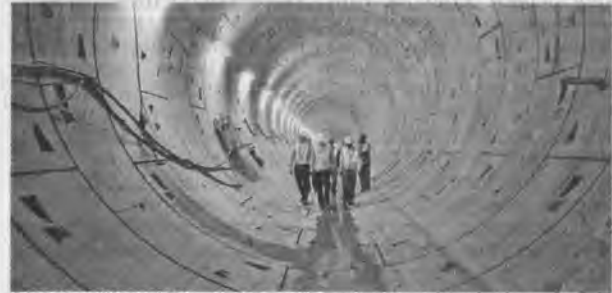
Metro rail workers at the underground station near Pachaiyappa's college in Chennai.
